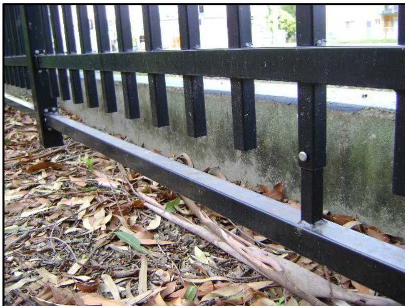
Picture 6.4: Type 1 Security Fencing with infill bar
